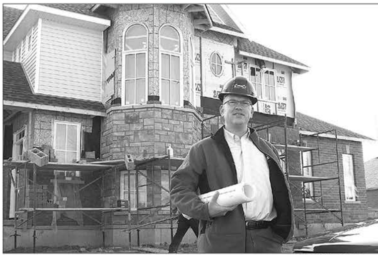
Ken Dantzer of Caraco Development Corp. stands in front of the energy-efficient home under construction on Crossfield Avenue. "There are people looking for this, but the majority of people are cost-conscious," Dantzer says.
